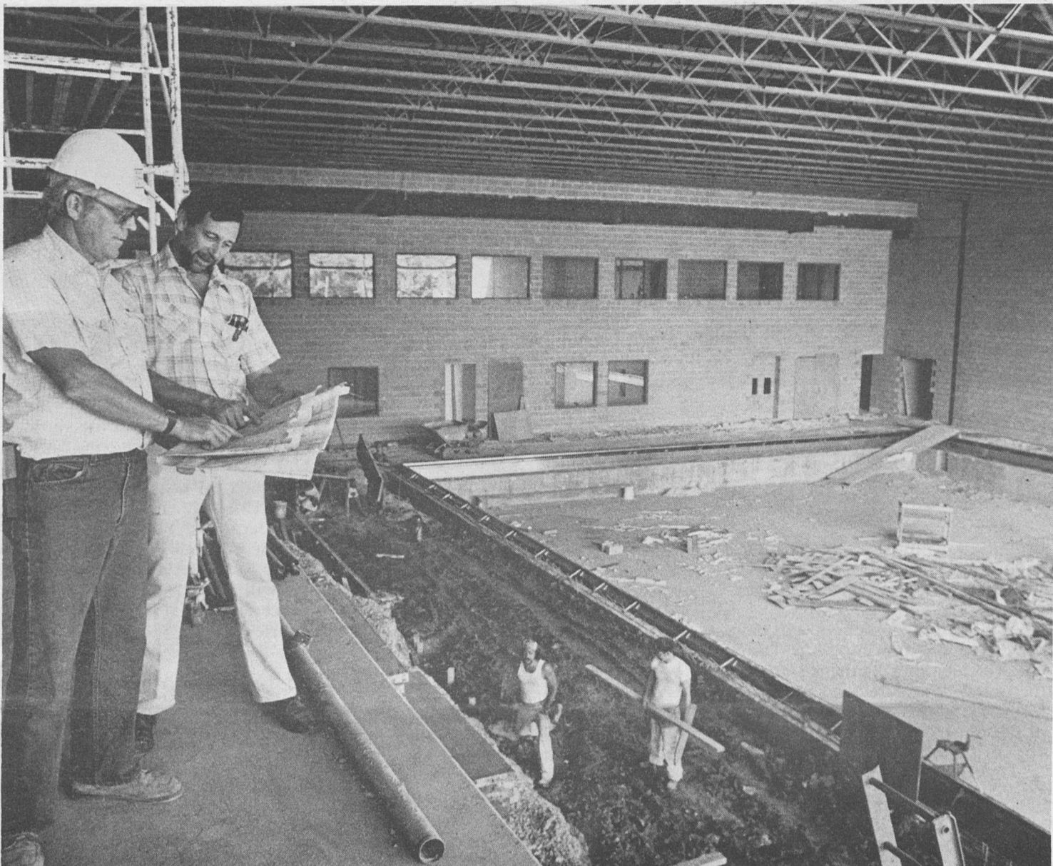
Poolside. Ray Schrader (left), projects superintendent for Kloester Construction Co., and Jack Reuter, construction representative for WU, review plans for the swimming pool being built as part of the first major renovation and expansion of the University's sports and recreation facility in more than 50 years. When completed in spring 1985, the heated, olympic size pool will be open to students, faculty and staff. In addition to eight swimming lanes, the pool will feature a diving area with one three-meter spring board and two one-meter spring boards.
